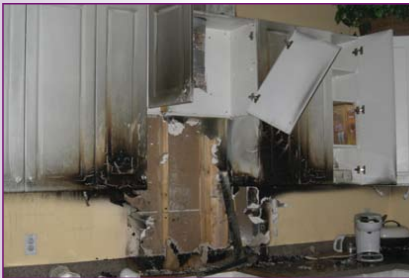
In October, our emergency shelter experienced a fire which destroyed the kitchen; smoke and water damaged the rest of the shelter. By December, Donna Lynne Custom Homes had led the way completing the renovation of the shelter.
